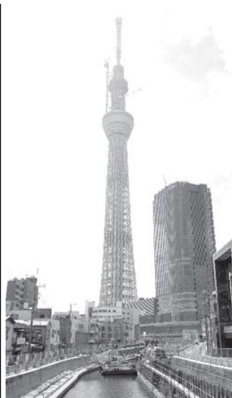
The under-construction "Tokyo Sky Tree" tower is seen in Sumida, Tokyo, Japan, on 8 June, 2010. According to the operator, the new tower will open on 22 May, 2012. "Tokyo Sky Tree" tower, with a height of 634 meters, is the world's highest self-standing tower.—XINHUA
