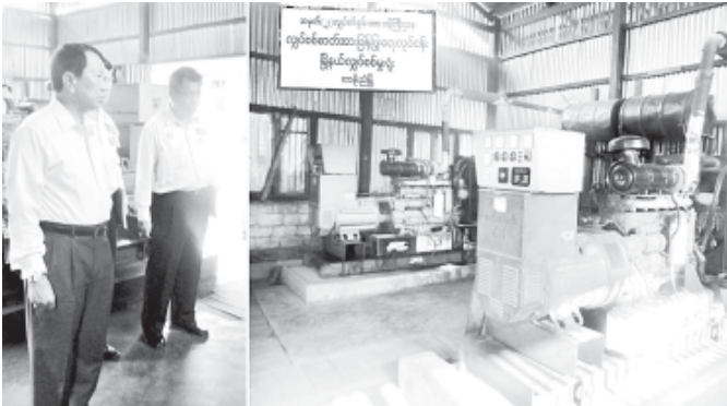
Union Minister for Electric Power No. 2 U Khin Maung Soe inspects two 150-KVA diesel generators in Tamoeyne.—MNA
