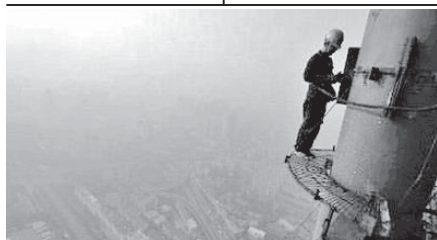
A labourer works on a steel structure at a financial building construction site, as the cityscape is seen amid smoke from burning straw, in Hefei, Anhui on 3 June, 2011. Growing evidence that China's roaring economy is starting to slow has fed an investor debate about whether the world's growth engine is gently easing or headed for a sharp downturn.—INTERNET
