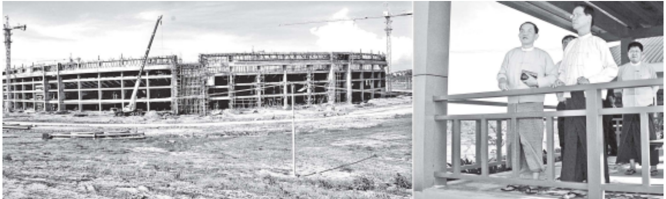
Vice-President of the Republic of the Union of Myanmar Dr Sai Mauk Kham inspects construction of Zabuthiri Advanced Sports Complex in Nay Pyi Taw Zabuthiri Township.—MNA
