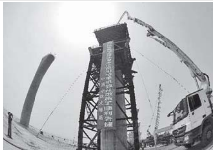
Photo taken on 17 May, 2011 shows construction site of the Jiaxing-Shaoxing Bridge in Hangzhou, east China's Zhejiang Province. The Bridge, which is designed to join Jiaxing and Shaoxing cities of east China's Zhejiang Province across the Hangzhou Bay, will be put into operation in 2012. It is expected to halve the journey between Shaoxing and the economic hub Shanghai to 1.5 hours by then. Currently, 130 piers have been erected and the bridge deck pavement is about to start.—XINHUA
