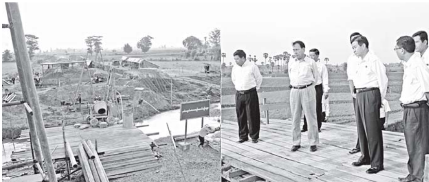
Union Minister for Rail Transportation U Aung Min views construction of Nawin Creek Bridge near Byaingin Village in Tatkon Township.— MNA
