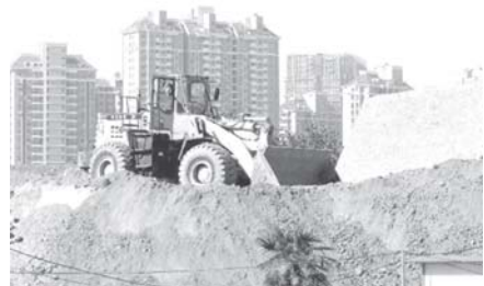
A tractor shovel is seen at the construction site of the rebuilding work on a 3,600-year-old city wall in Zhengzhou, central China's Henan Province, on 13 May, 2011. The restoring work has triggered controversies in China.— XINHUA
