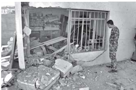
An Iraqi policeman inspects the damage to a house belonging to a lawmaker in Kirkuk, 290 kilometres (180 miles) north of Baghdad, Iraq, on 12 May, 2011. An Iraqi lawmaker from the Sunni-backed Iraqiya bloc escaped an assassination attempt Thursday in the ethnically mixed city of Kirkuk.
