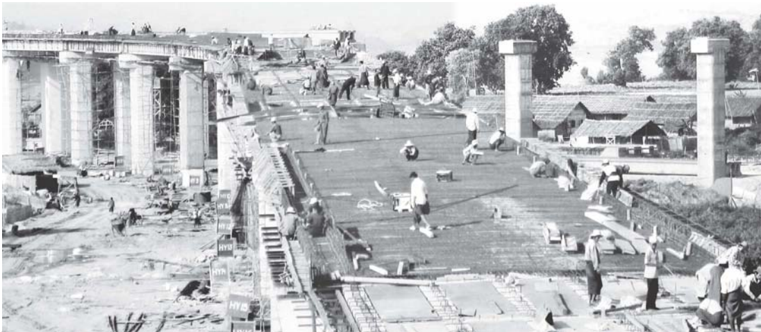
Concrete works being placed on approach road (motor road) of Ayeyawady Bridge (Malun) on Migyaungye bank.
