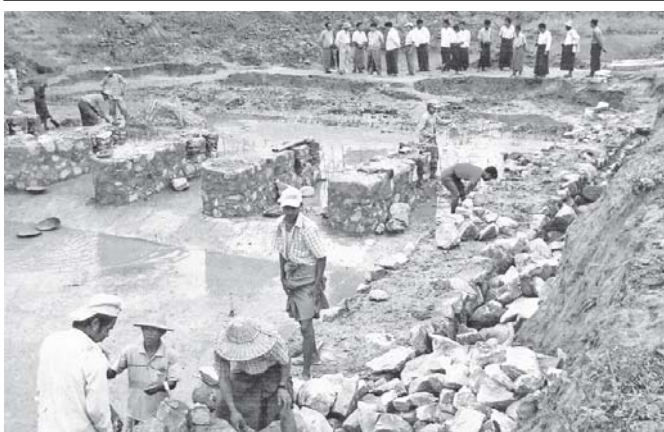
Nay Pyi Taw Council member U Than Aung looks into Kyarku Dam being built by Dekkhinathiri Township Irrigation Department near Hsesu village in Kyuntatpat village-tract. (News reported)—MNA
