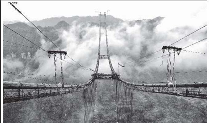
Photo taken on 2 May, 2011 shows the Aizhai suspension bridge under construction in western Hunan Province, central China. The steel truss girder structure has the country's longest suspension bridge main span of 1,176 meters.—XINHUA
