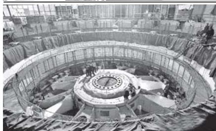
Technicians install the No 30 turbine at Three Gorges' underground power station in Yichang, central China's Hubei Province, 26 April, 2011. The No 32 turbine of the hydropower project started its water filling test on Tuesday. It is expected to be put into operation in May of 2011. Three of all the six underground turbines are scheduled to be put into operation before the flood season of this year.—XINHUA
