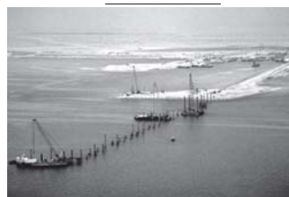
An aerial view of the construction progress on oil drilling pads in the Gulf off Manifa Bay, a natural shallow water harbour about 180 kms northwest of Dhahran.
