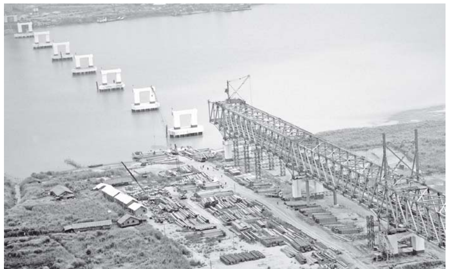
Photo shows an aerial view of Ayeyawady Bridge (Nyaungdon) project in Nyaungdon Township—MNA
