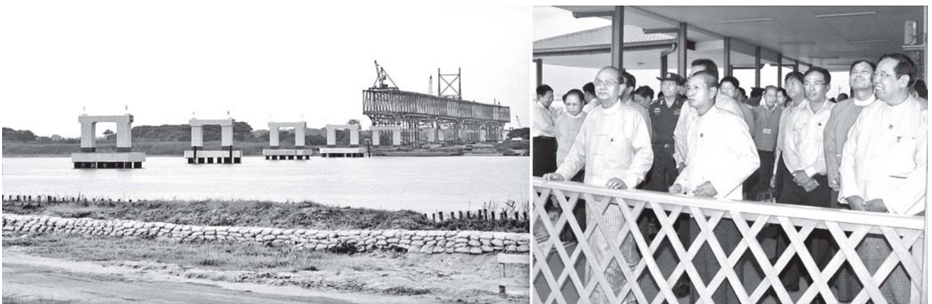
President U Thein Sein inspects steel truss installation at Ayeyawady Bridge (Nyaungdon).—MNA
