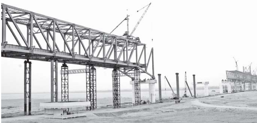
Photo shows completion of installation of steel truss of the bridge on Letpanchepaw bank.—MNA
