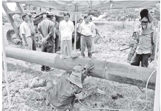
Union Minister for Energy U Than Htay inspects construction of Pyawbwe-Pyinmana-Yeni-Taungphila natural gas pipeline.—MNA
