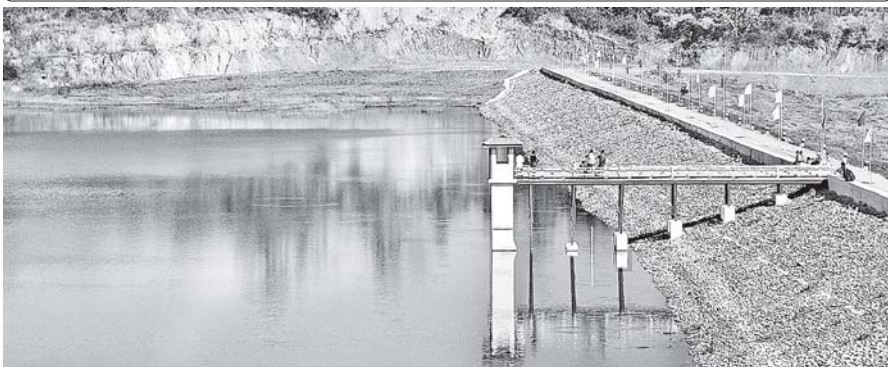
ThanU Chauk Dam being constructed by Magway Region Irrigation Department in Kyaukhtu Township, Gangaw District, Magway Region.—MNA
