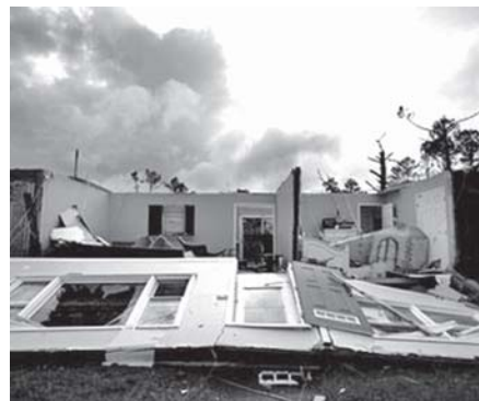
A tornado flattened most of this home in the LaGrange subdivision, 16 April, 2011 in Fayetteville, NC. Homes and businesses were badly damaged Saturday by a severe storm system that whipped across North Carolina, bringing flash floods, hail and reports of tornadoes from the western hills to the streets of Raleigh.—INTERNET
