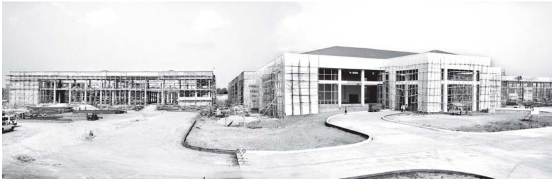
Photo shows progress of National Museum (Nay Pyi Taw) on Yazathingaha Road in Zabuthiri Township of Nay Pyi Taw District.—MNA
