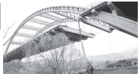
Photo taken on 12 April, 2011 shows the site of a bridge collapse accident in the suburbs of Korla City, northwest China's Xinjiang Uygur Autonomous Region. A bridge on National Highway 314 collapsed at 5:30 am Tuesday. There were no reports of any casualties so far. —XINHUA
