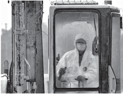
A worker wears protective gear as he operates excavator at an area that was damaged by the March 11 earthquake and tsunami, which is about 20km (12 miles) from the damaged Fukushima nuclear power station, in Minamisoma, Fukushima Prefecture, on 9 April, 2011. INTERNET
