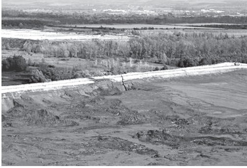
Picture taken in 2010 shows cracks on the north side of the reservoir wall of the aluminium plant near Ajka, some 160 kms southwest of Budapest.
