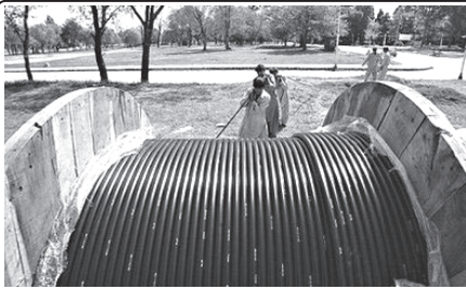
Workers roll a fibre-optic cable. Georgian police arrested a 75-year-old woman who single-handedly cut off Internet connections in Georgia and neighbouring Armenia, the interior ministry in Tbilisi said on Wednesday.
