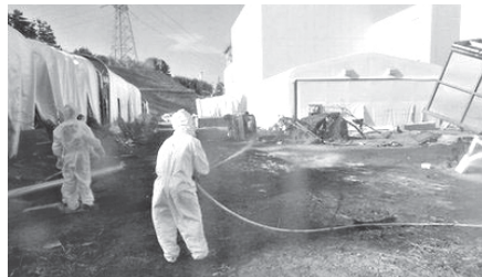
This handout picture, taken by Tokyo Electric Power Co (TEPCO) on 1 April, shows workers spraying resin on the ground near the reactor buildings. Three weeks after watching a massive wave smash into the Fukushima nuclear plant, Hiroyuki Kohno is heading back to the disaster zone to join crews struggling to avert a meltdown.—INTERNET
