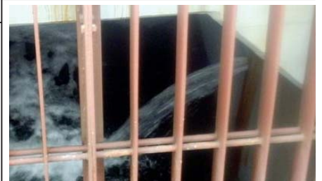
In this 2 April, 2011 photo released by Tokyo Electric Power Co via Kyodo news, leaking radioactive contaminated water drain through crack of a maintenance of Fukushima Daiichi nuclear power plant in Okumamachi, Fukushima Prefecture, northeastern Japan.—INTERNET
