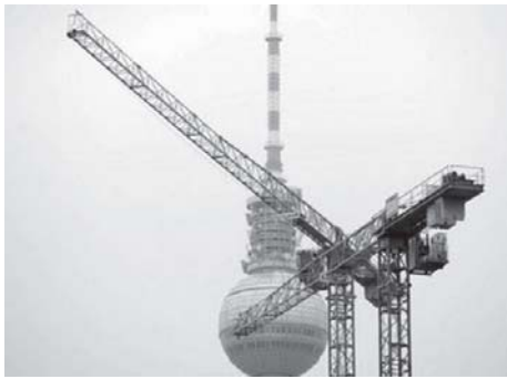
Cranes active on a building site operate near Berlin's landmark TV tower, 2010. Germany's Ifo indicator of business confidence in Europe's top economy fell in March for the first time since May.
