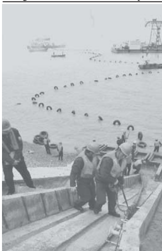
Workers drag a submarine cable onshore in Chengsi Island, Zhoushan City, east China's Zhejiang Province, on 16 March, 2011. XINHUA
