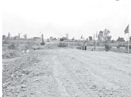
Minister for Rail Transportation U Aung Min inspects Nay Pyi Taw-Hsinthe (Tatkon)-Pinlaung Railroad construction.—MNA
