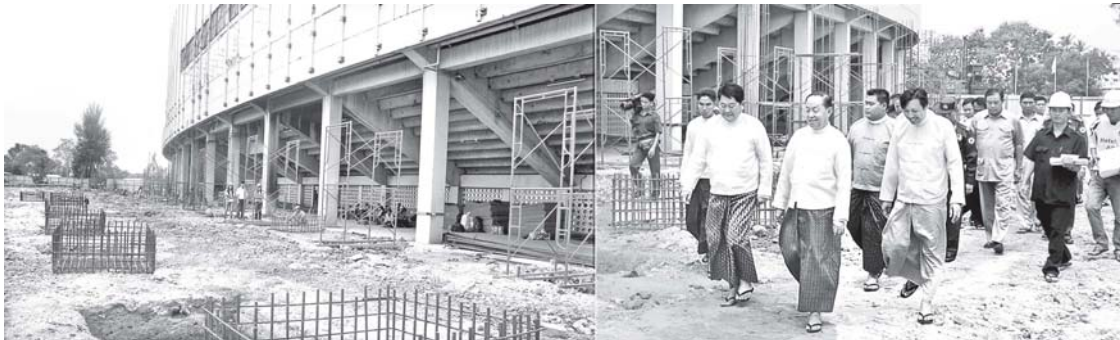
Secretary-1 of the State Peace and Development Council Thiha Thura U Tin Aung Myint Oo inspects extended construction of football stand at Youth Training Centre (Thuwunna).—MNA
