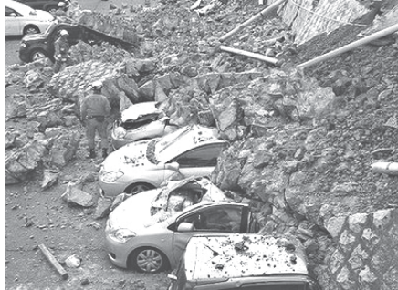
Vehicles are crushed by a collapsed wall at a carpark in Mito city in Ibaraki prefecture after a massive earthquake rocked Japan. The strongest quake on record to hit Japan Friday unleashed a terrifying 10-metre tsunami that claimed hundreds of lives, with a nuclear plant and petrochemical complex among multiple sites set ablaze.
