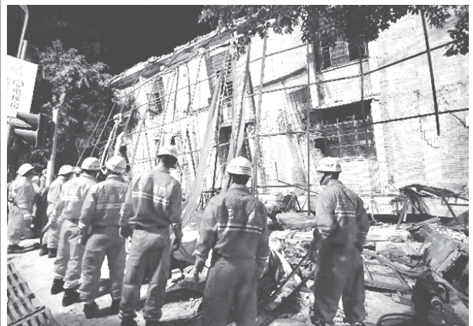
Firefighters dismantle a damaged house after a 5.8-magnitude earthquake hit Yingjiang County in southwest China's Yunnan Province, on 11 March, 2011. A 5.8-magnitude earthquake jolted Yingjiang County Thursday noon, killing at least 25 people and injuring 250 others.
