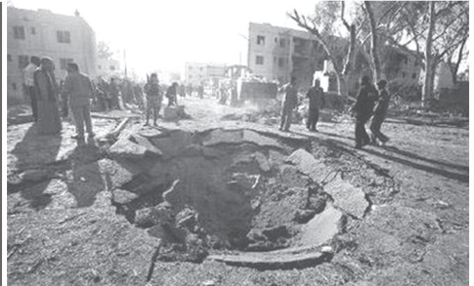
A crater is left in a pavement after a suicide truck bomb attack in Baiji recently.—INTERNET
