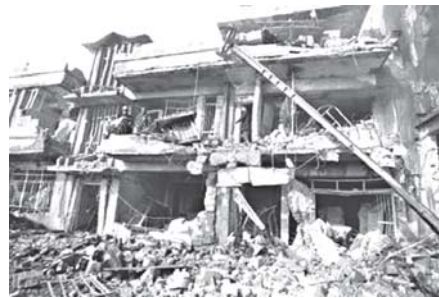
Civil defence personnel inspect a damaged building after a bomb attack in Kirkuk, some 250 km (155 miles) north of Baghdad recently. Three car bombs killed four people and wounded 20 others in Iraq's oil-rich northern City of Kirkuk on Wednesday, police and hospital sources said. INTERNET
