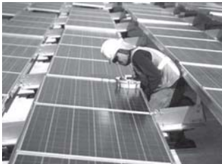
A worker installs solar panels atop a government building in Colorado. The United States, taking the helm of the APEC forum, hopes to spur green growth in the Asia-Pacific region by knocking down trade barriers on environmental goods, a senior official has said.
