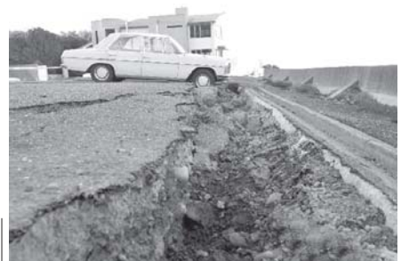
A splitted road is seen in east suburb of Christchurch after the earthquake, on 1 March, 2011. Police began to evacuate residents in east suburb of Christchurch as cracks emerged in the hill at the area.
