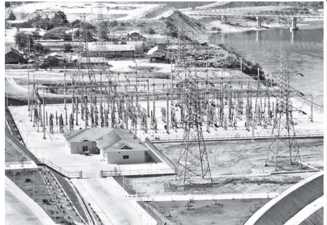
The switchyard of Yeywa Hydropower Plant.
