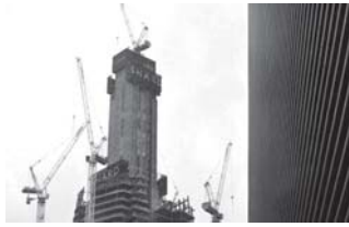
Construction work continues on a 'The Shard', a new building in central London, seen here in October.
