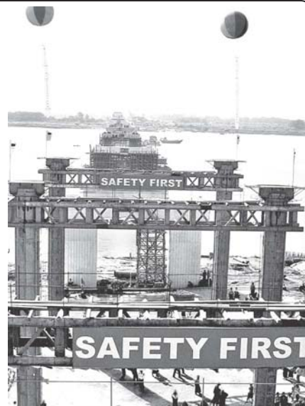
Pillars of Ayeyawady Bridge (Nyaungdon) are ready to be installed with iron frames.
