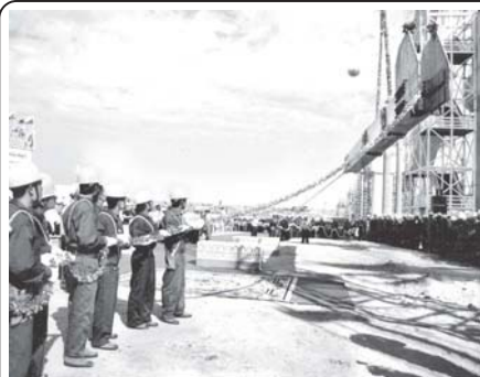
Myanmar workers participate in lifting first iron frame onto Ayeyawady Bridge (Nyaungdon).
