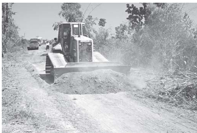
Kyetyin-Gaungbwa-Letpan Inter-Village Road being built by Shwetaung Co with the use of heavy machinery.
