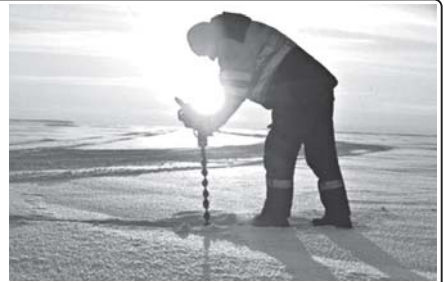
A worker measures the thickness of the ice along Estonia's ice road on 17 February. The 26.5 kms ice road in western Estonia, which links the mainland to the country's second largest island of Hiiumaa, is Europe's longest.
