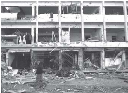
Afghan police officers and locals inspect a damaged hotel building near a police headquarter which was attacked on Saturday by Taliban militants in Kandahar, south of Kabul, Afghanistan, on 15 Feb, 2011.
