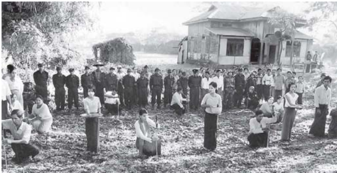
Head of Labutta Township Information and Public Relations Department, Chairman of Bopyae Village-tract Peace and Development Council U Thein Tun, and community elders drive stakes for construction of Bepauk Village Library on 13 February.—TOWNSHIP IPRD
