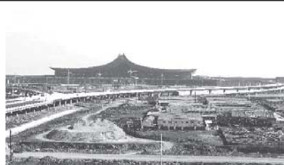
Photo taken on 10 Feb, 2011 shows the construction site of the new airport of Kunming, capital of south China’s Yunnan Province. The investment of the new airport of Kunming has reached 14.26 billion RMB yuan, 75 percent of the project’s total budget.
