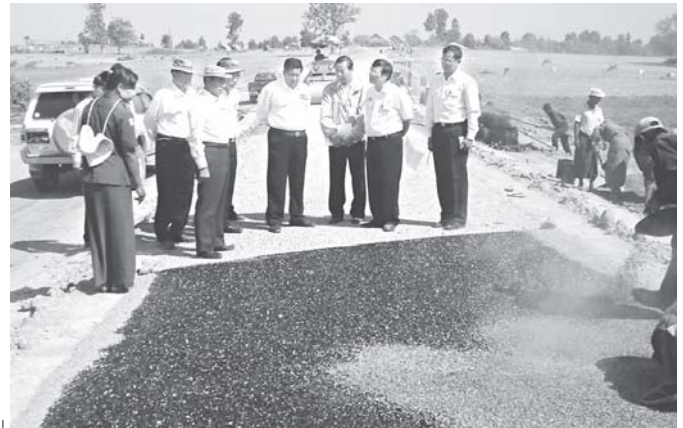
Minister for Construction U Khin Maung Myint looks into tarmacking of Koebin-Thagara Road.—CONSTRUCTION
