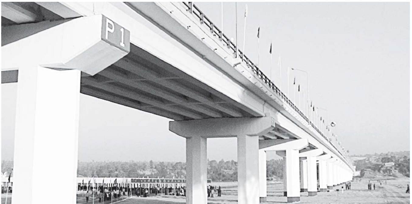
Photo shows Daungnay Creek Bridge, 255th facility in the nation, on Yangon-Pyay-Magway-Mandalay Road in Magway Township.—MNA
