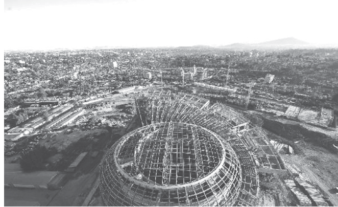
Photo taken on 28 Jan, 2011 shows the new African Union (AU) Conference Centre in Addis Ababa, Ethiopia. The construction process of new AU Conference Center by China had finished the sealing of roof structure and began the internal decoration. The project will be completed at the end of 2011.
