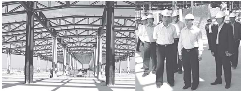
Minister U Thein Swe oversees construction of Nay Pyi Taw International Airport.
