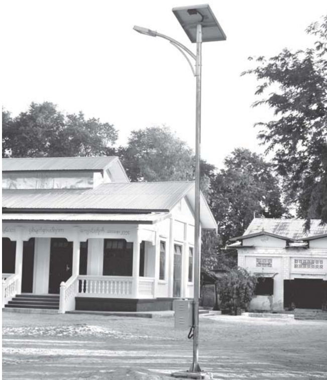
A solar lamp post installed with solar panel, bulb and energy control system in Ywathaya Village.
