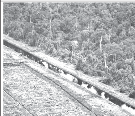
Excavators are seen constructing drainage canals and roads on a logged area of the Kerumutan peat swamp forest in Sumatra. A series of deals between India and Indonesia worth $15 billion includes cooperation in infrastructure, manufacturing and natural resources.
