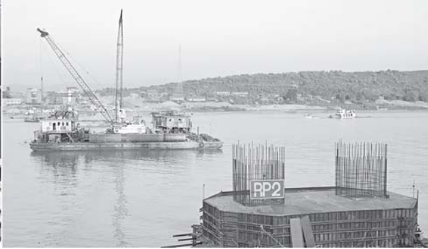
Maj-Gen Myint Soe of Ministry of Defence inspects progress of Yadana Theinga Bridge near Kyaukmyaung-Nwenein Village in Shwebo Township. (News on page 1)
