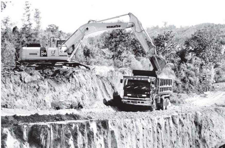
An excavator and a delivery truck carry out groundwork to build a section of Koebin-Thagaya Road.
