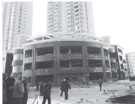
Photo taken on 17 Jan, 2011 shows the accident site in Jilin City, northeast China's Jilin Province. An explosion occurred inside a building in the city early Monday, causing three people dead and nearly 20 people injured.
