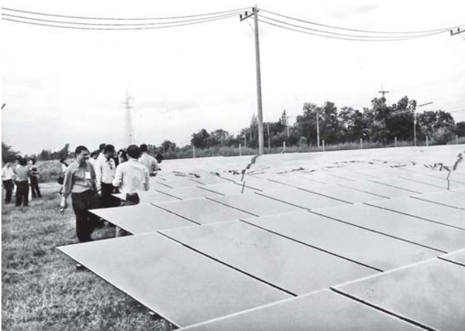
The solar panel field near Hua Hin, Thailand.
