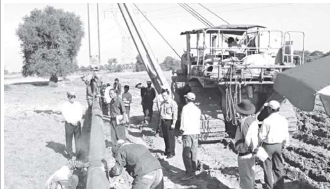
Minister for Energy U Lun Thi inspects welding work and laying of natural gas pipelines at Pyawbwe-Tatkon section.—MNA
