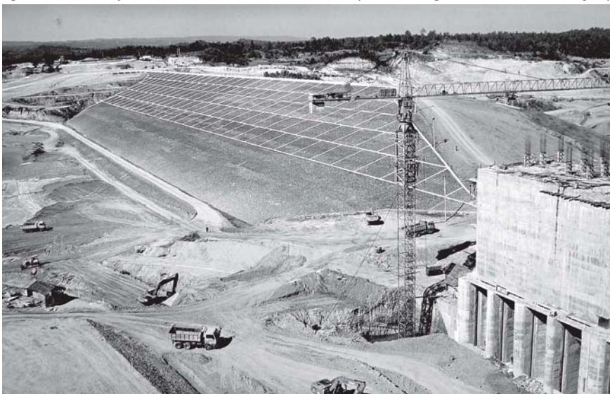
Earth work of Kyee-Ohn Kyee-Wa Multi-Purpose Dam Project is being undertaken with the use of machinery near hydro power station.
