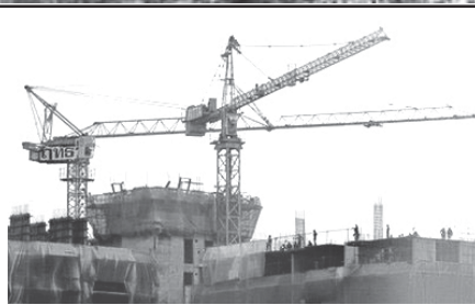
A commercial facility is seen under construction in central Bangkok. China will build a "commercial city" in Thailand worth $1.5 billion that will allow traders to re-export Chinese-made goods and avoid costly tariffs, state media said Thursday.
