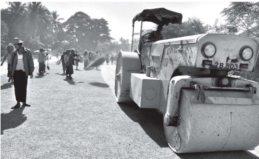
Quality control is one of the top priorities in implementing four-lane Pyinmana-Taungnyo Road Project.
