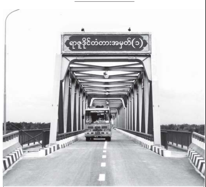
Yazudaing Bridge No. 1, 1955 feet long, built in Mawlamyinegyun Township, ensures better transport in Ayeyawady Region.
