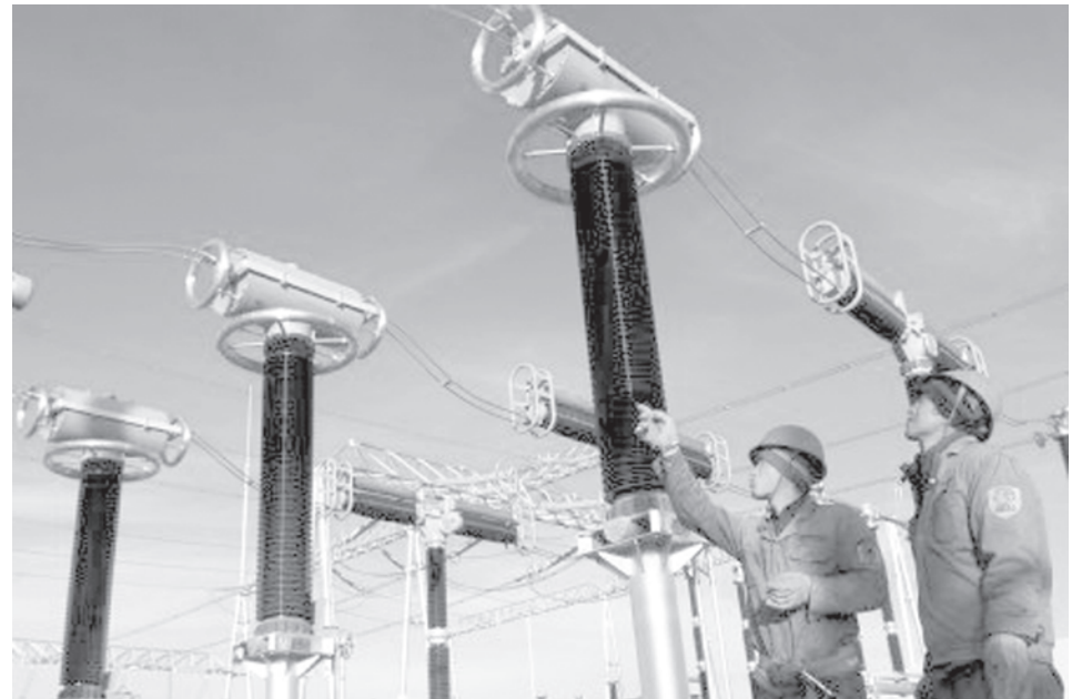
Workers debug the equipment at the wind power base in Jiuquan City, northwest China's Gansu Province, recently. The Jiuquan wind power base achieved the landmark capacity as the result of the installation of a 200-megawatt wind power unit in Yumen, a city under the jurisdiction of Jiuquan.—INTERNET
