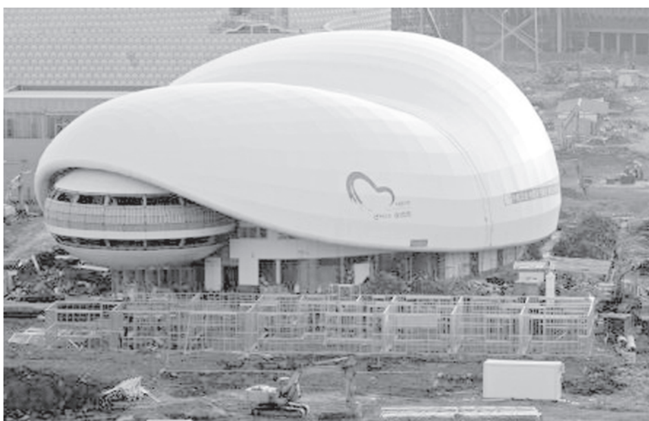
The photo taken on 26 Dec, 2009 shows the China Aviation Pavilion under construction for 2010 Shanghai World Expo in the Puxi zone of World Expo Park in east China's Shanghai Municipality. —XINHUA
